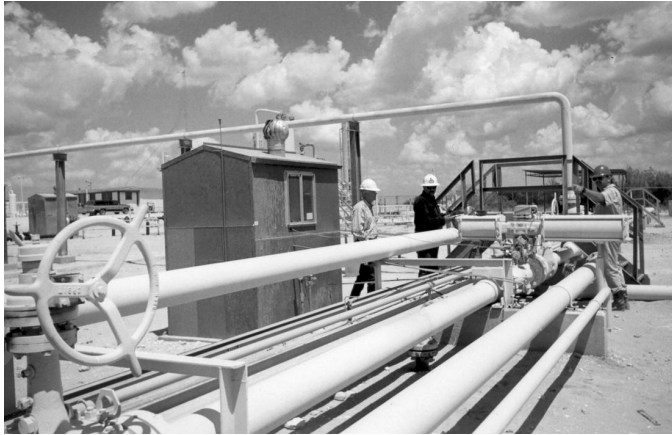
Figure 3-4 A metering station must be properly installed and maintained to provide accurate measurement.
