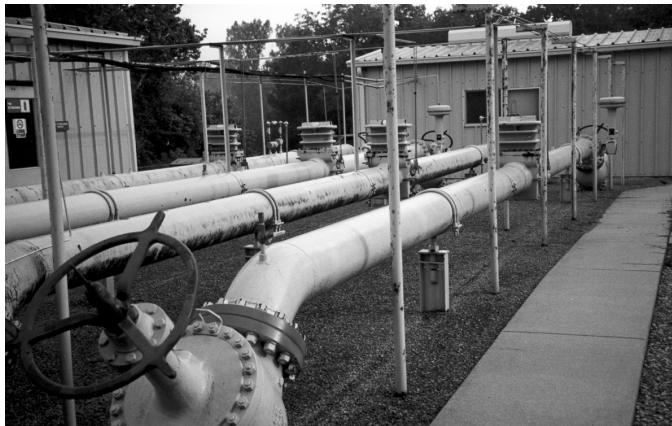
Figure 3-2 Typical meter and regulation station.
