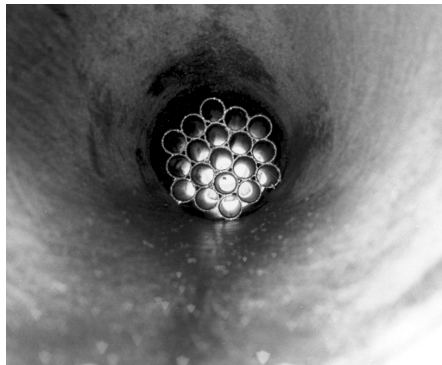
Figure 7-4 Swirl must be eliminated for accurate flow measurement. Note swirl pattern on pipe wall.
