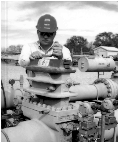
Figure 5-11 Meters and meter tubes must be properly maintained for accurate flow measurement.
