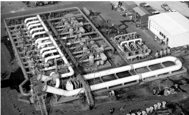
Figure 3-6 Large pipe prover for liquid turbine meters.
