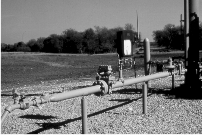
Figure 13-2 Typical orifice meter installation.
