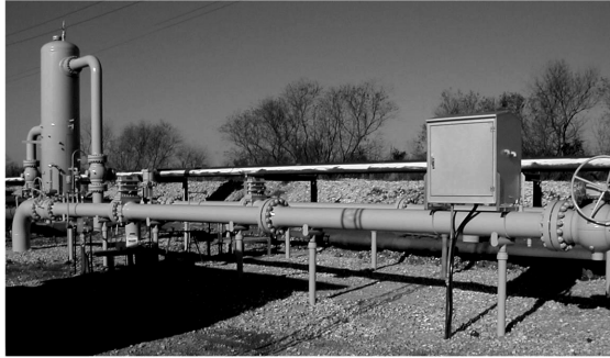
Figure 5-14 A well designed metering station properly installed and maintained represents a good value whose reliable measurement accuracy will maximize the return on investment.
