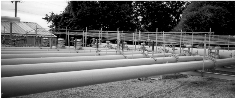
Figure 5-6 Good design calls for long, straight meter-tube lengths for the most accurate flow measurement with minimum uncertainty.
